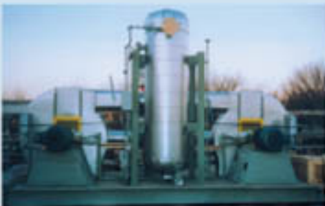
This Aqueous Exhaust Recirculating AFCU Skid is capable of vaporizing 550 lbs/hr of aqueous ammonia.
