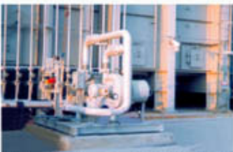
This Anhydrous AFCU Skid is operating at a 240 MW merchant power plant in Texas.
