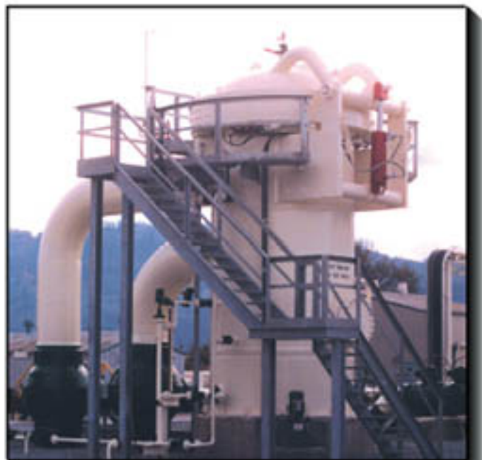
This Absolute Separator is installed in a metering station in Canada. Its 99" ID housing utilizes a full diameter, quick-opening closure. This system is fitted with an 'On-line Monitoring System' to continually measure coalescing-filter element permeability.
